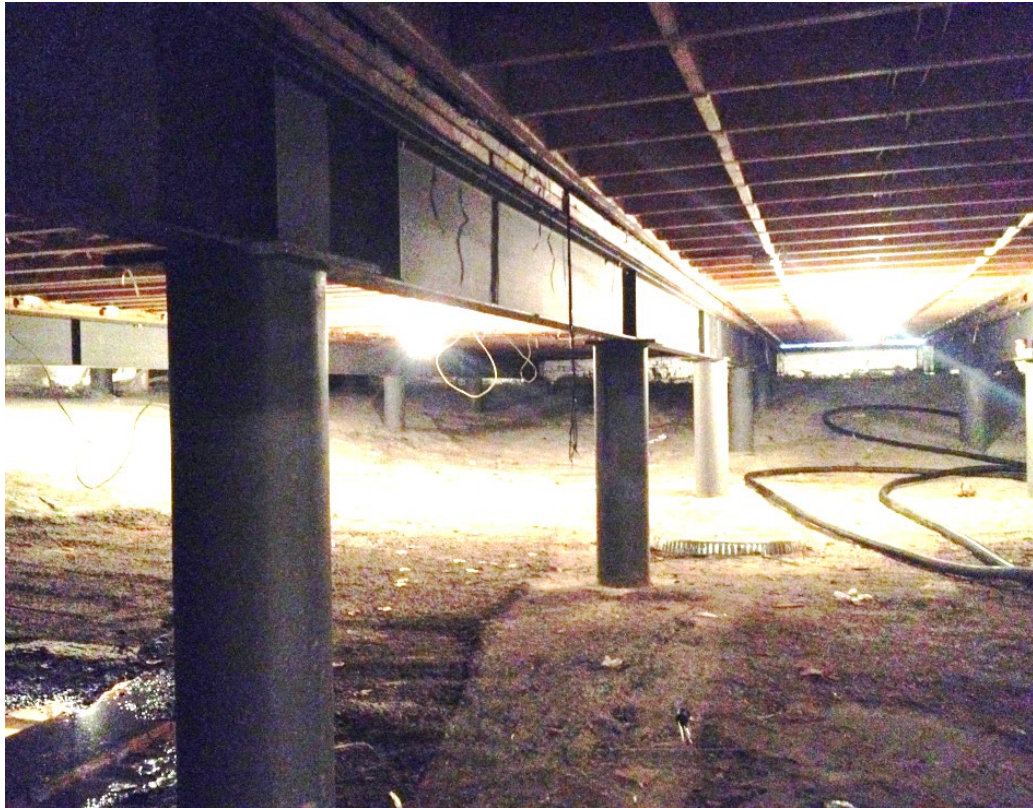
Crawlspace: Typically utilities would be run below the buildings.
