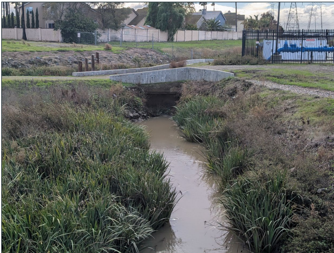
Figure 2: Erosion at Drainage Ditch Crossing
