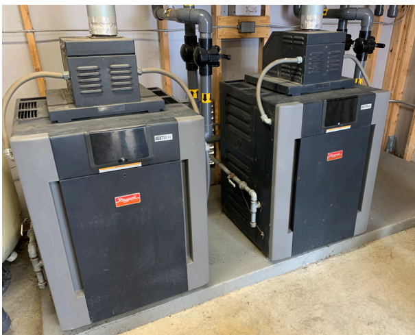
Figure 3.5: Natural Gas Pool Heaters
