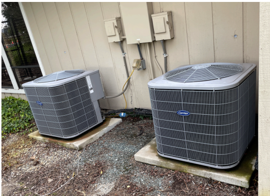
Figure 3.2: Outdoor Air Conditioners serving the Community Center
