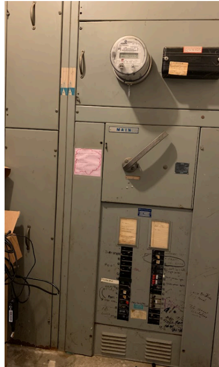
Main Electrical Switchgear Panel - Community Center
