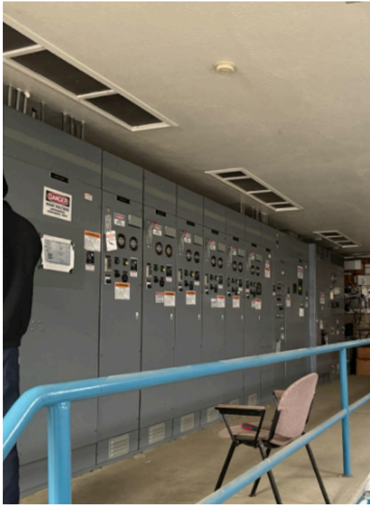
Main Electrical Switchgear Panel & Meter - Willow Lake Treatment Plant
