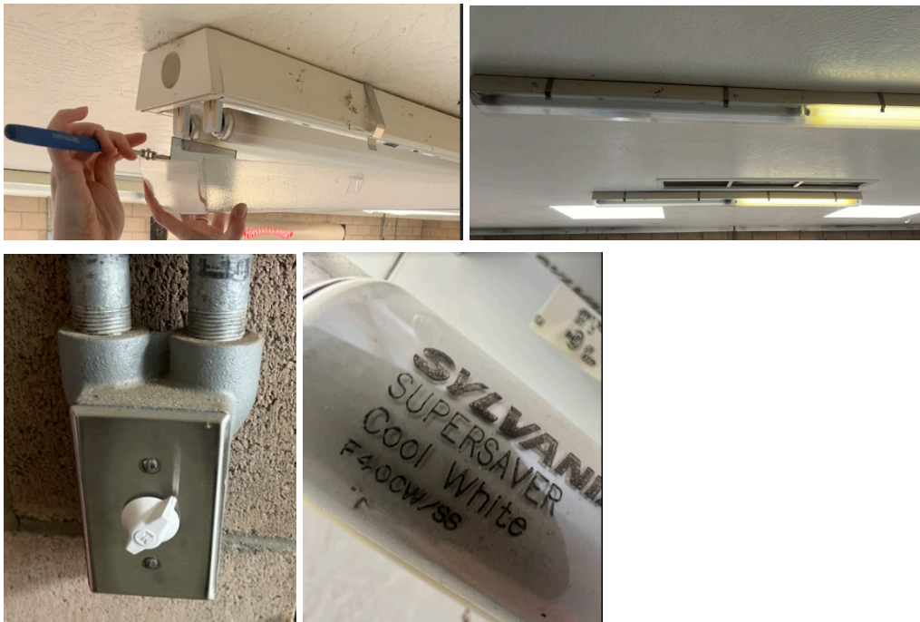
Figure 3.7: Willow Lake WTP - Pump Station Lighting
