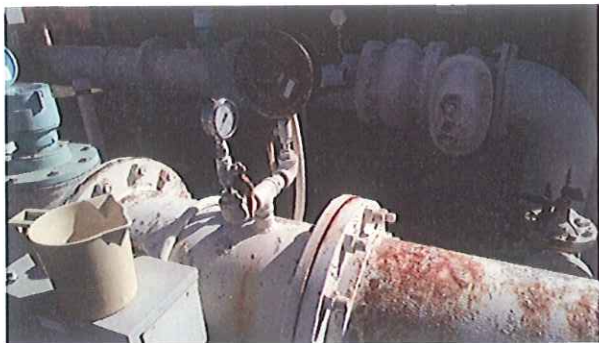
Corroded HP switch and mixed piping
