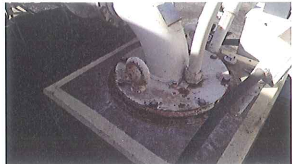
Corroded pump baseplate
