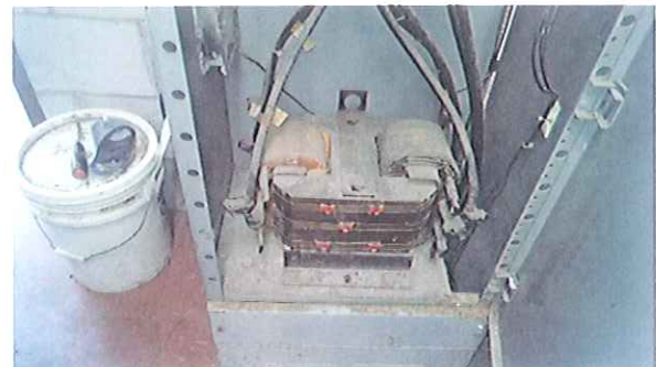
Old electrical switchgear
